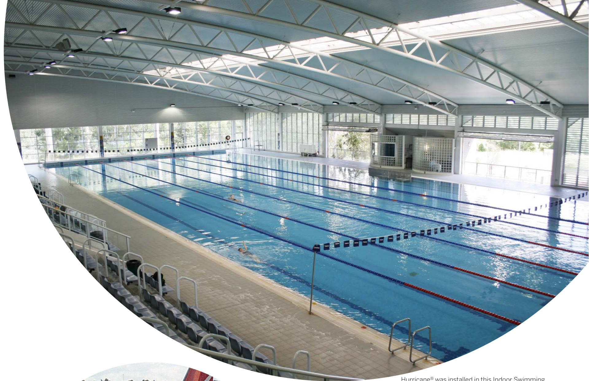
Hurricane® was installed in this Indoor Swimming Centre to reduce condensation and humidity.
